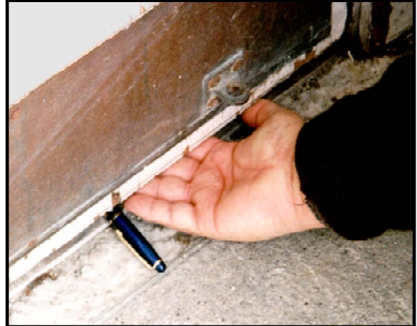
Figure 10: This gap at the bottom of the door is large enough to allow rat and mouse access to the building. Installation of a door sweep would exclude rodents.
