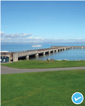
McNear's Beach Park pier repair underway, and entryway repaving completed , rebuilding key infrastructure.
