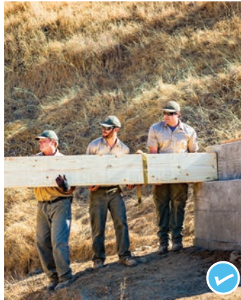
New bridge, 1,000 linear feet of trail, and habitat restoration in Loma Alta Preserve repaired an eroding portion of the Old Railroad Grade Trail known as "the Plunge."
